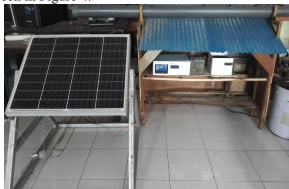
Figure 4. Solar Panel Implementation
